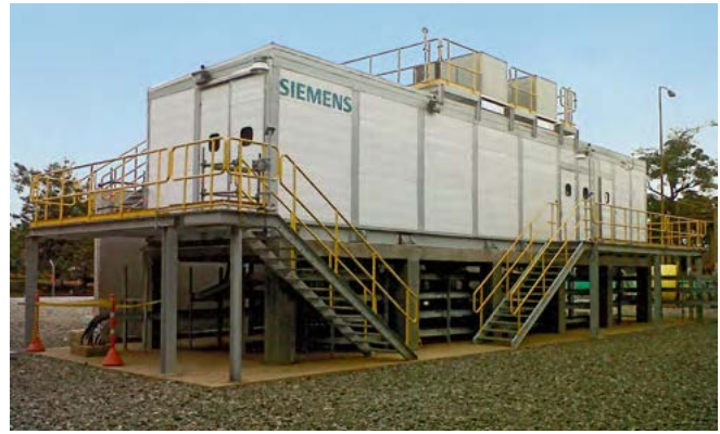
Fig. 2.4-6: E-house for mining in Columbia
