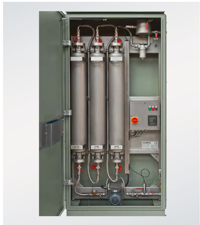
Fig. 5.13-5: Cabinet version of SITRAM DRY equipped with a control module
