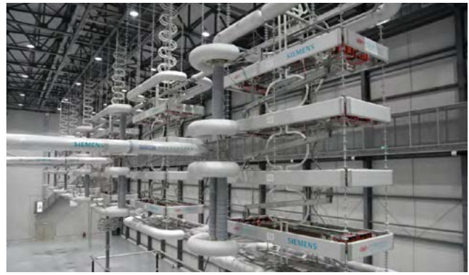
Fig. 2.2-5: UH voltage and power electronics – the thyristor valves are designed to operate at 800 kV voltage level. Yunnan-Guangdong, China
