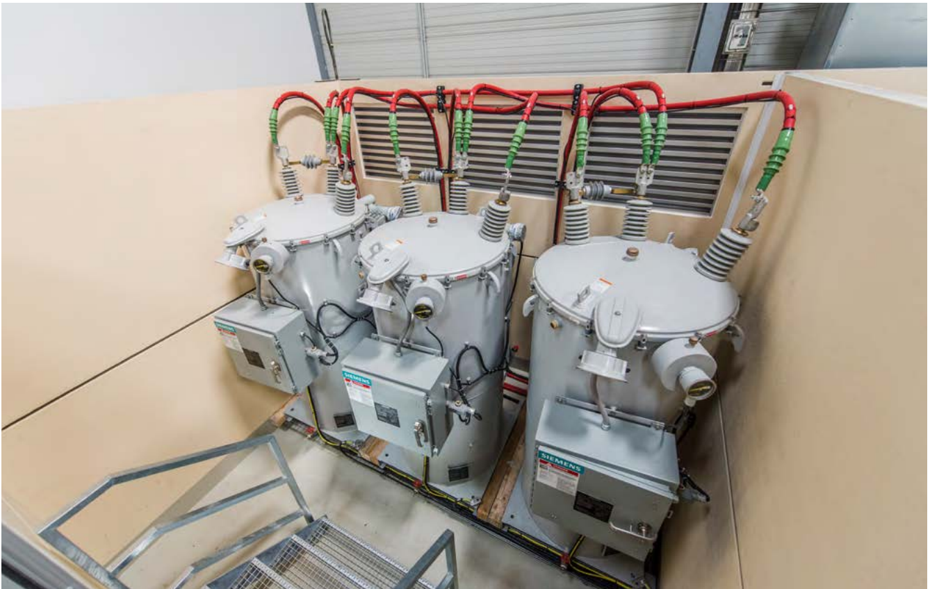
Fig. 5.11-4: In-phase voltage regulators, Niederstetten, Germany
