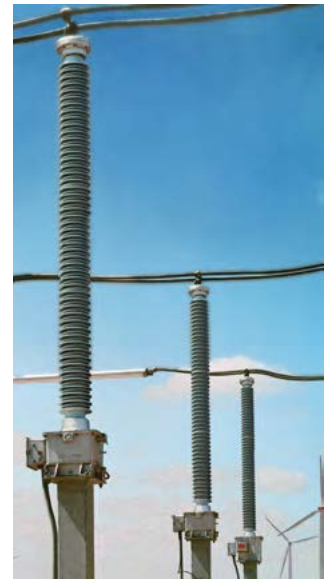
Fig. 4.2-20: 245 kV capacitor voltage transformers at Oncor substation (USA)
