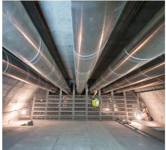
Fig. 2.2-51: Vertically installed GIL in Xiluodu, China
