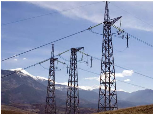
Fig. 4.2-3: 400 kV line in Bulgaria, NGLA solution realized with 3EL2
