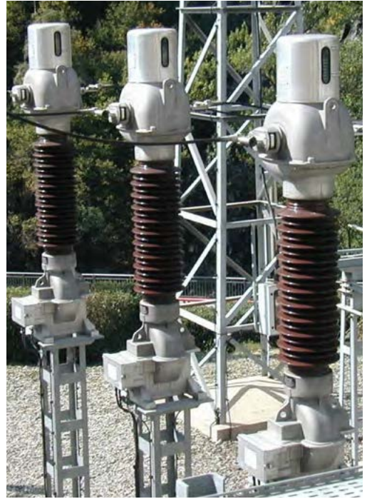
Fig. 4.2-18: 145 kV oil-immersed combined instrument transformer
