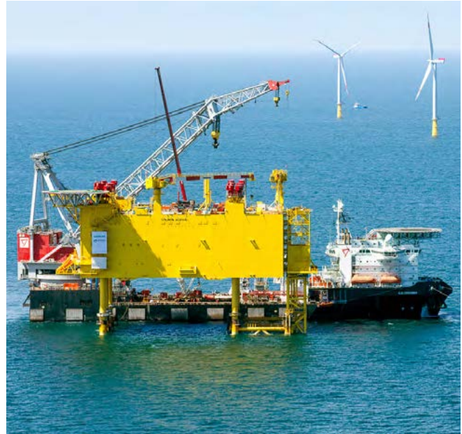
Fig. 2.2-37: SylWin 1, 864 MW HVDC PLUS, North Sea
