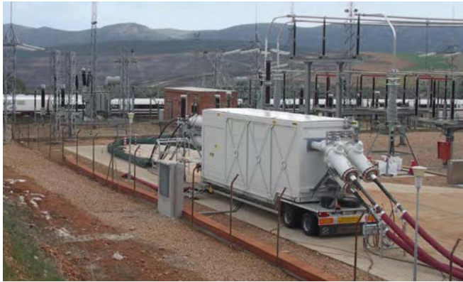
Fig. 2.4-13: 245kV Mobile substations with HV cable connection
