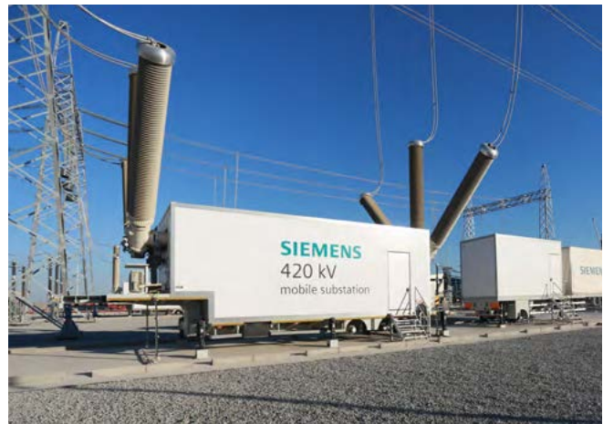
Fig. 2.4-24: world first 420kV mobile substation
