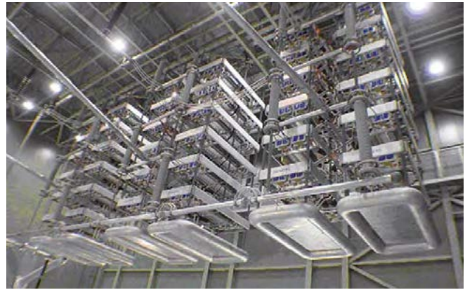
Fig. 2.2-2: Earthquake-proof and fire-retardant thyristor valves in 500 kV long-distance transmission in Guizho-Guangdong, China
