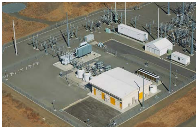
Fig. 2.2-21: Site view SVC PLUS in Australia
