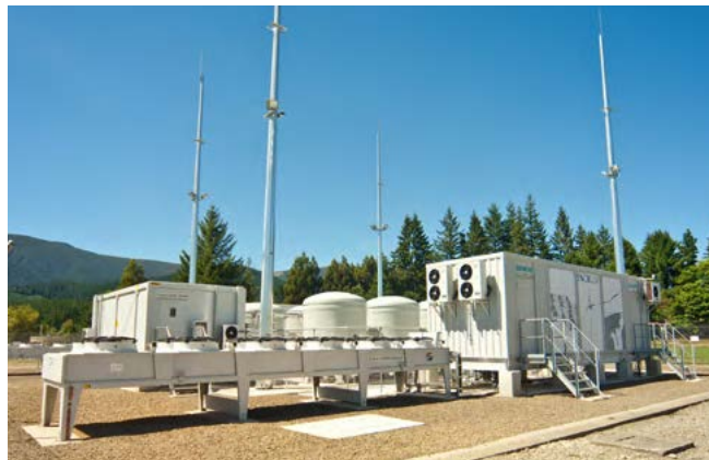
Fig. 2.2-20: SVC PLUS units in New Zealand
