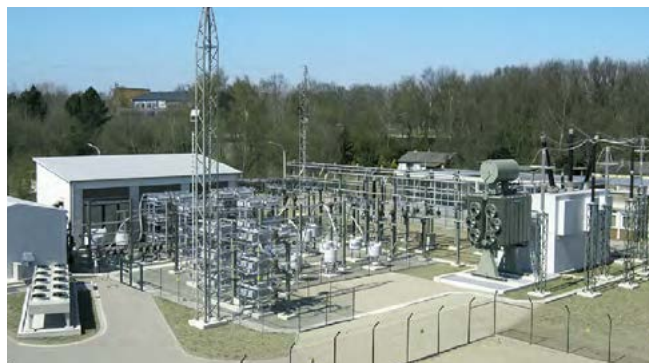
Fig. 2.2-19: Static Var Compensator (SVC) installation
