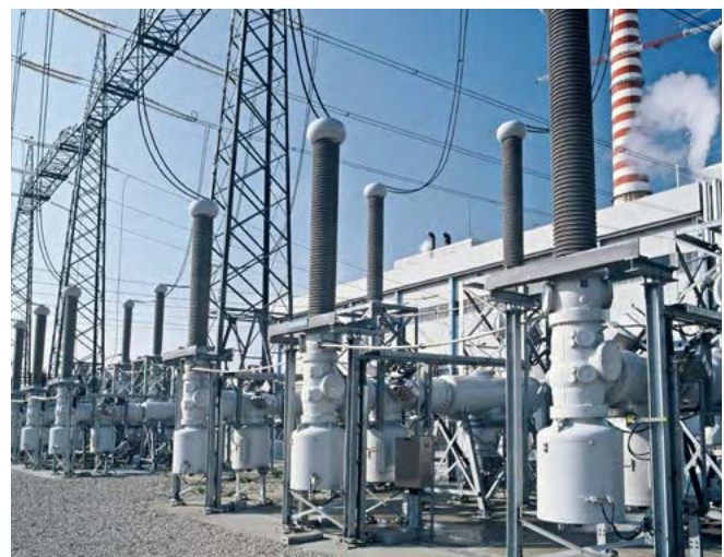
Fig. 6.2-10: Application in the high-voltage system
