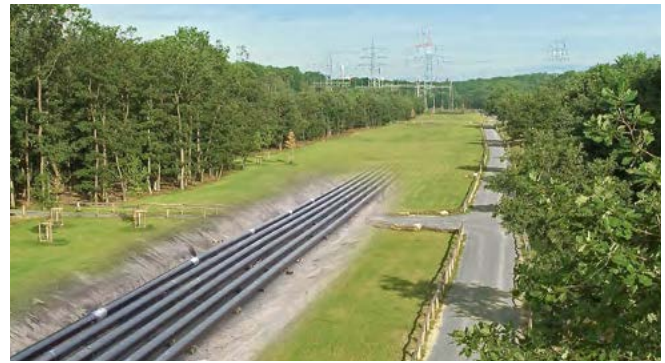
Fig. 2.2-47: Directly buried GIL
