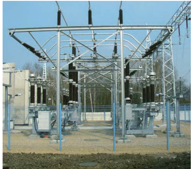
Fig. 3.1-26: H-arrangement with SIMOVER, 145 kV, Czech Republic
