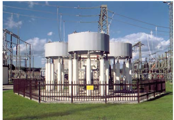
Fig. 4.2-35: Tertiary-connected shunt reactors
