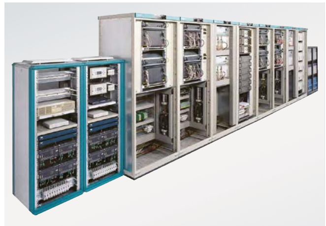
Fig. 2.2-17: The control and protection cubicles are intensively tested in the Siemens laboratories before they are shipped to site, assuring fast and smooth commissioning of the HVDC system
