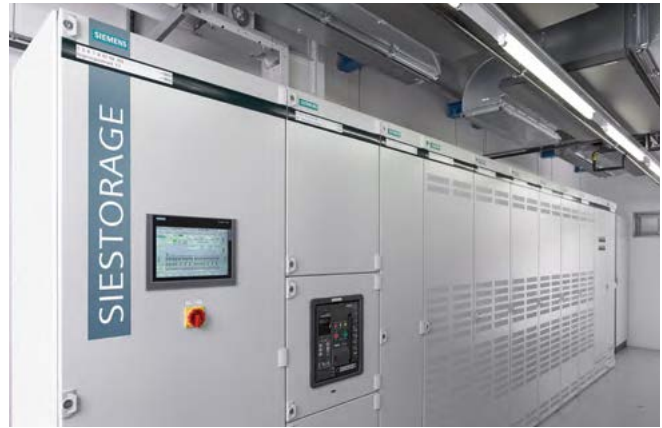
Fig. 2.3-16: SIESTORAGE system installed in an existing electrical building at the steel mill of the AMEH in Eisenhüttenstadt, Germany
