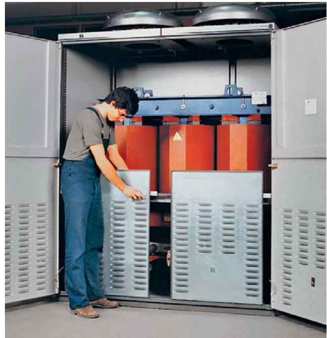
Fig. 5.11-10: GEAFOLE transformer in protective housing to IP20/40
