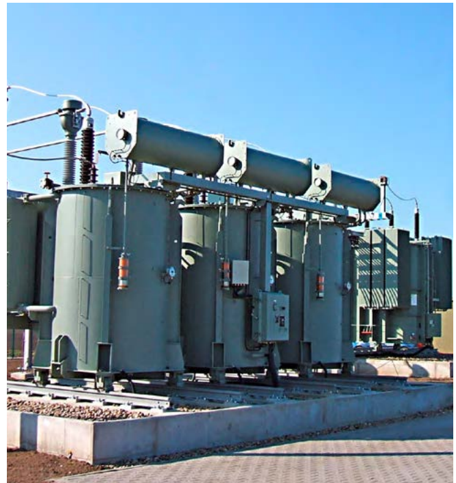
Fig. 4.2-38: Variable shunt reactor
