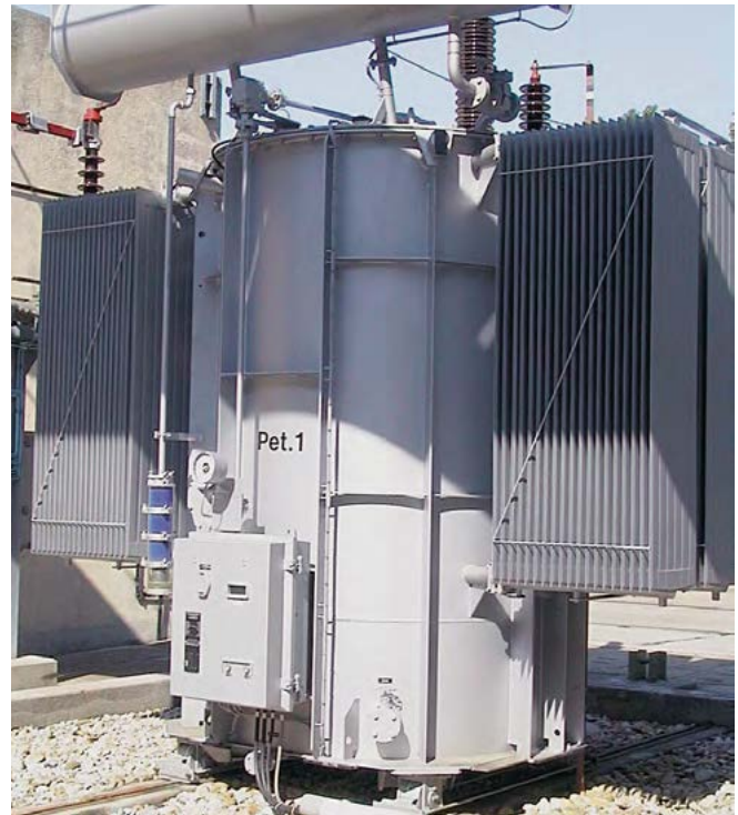
Fig. 4.2-37: Arc-suppression coil 110 kV
