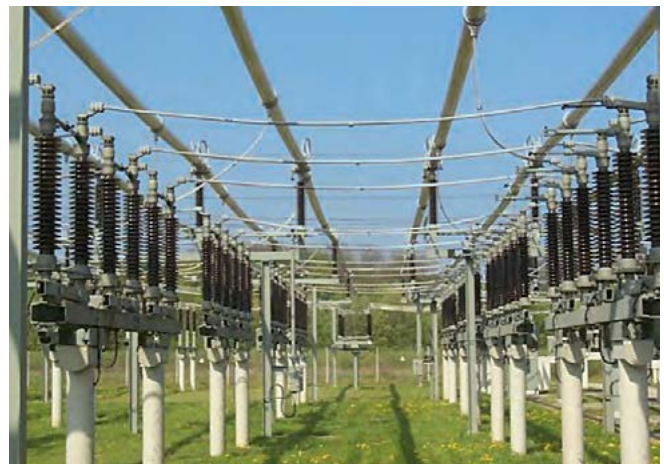
Fig. 3.1-14: Busbar disconnectors "in line", 110 kV, Germany
