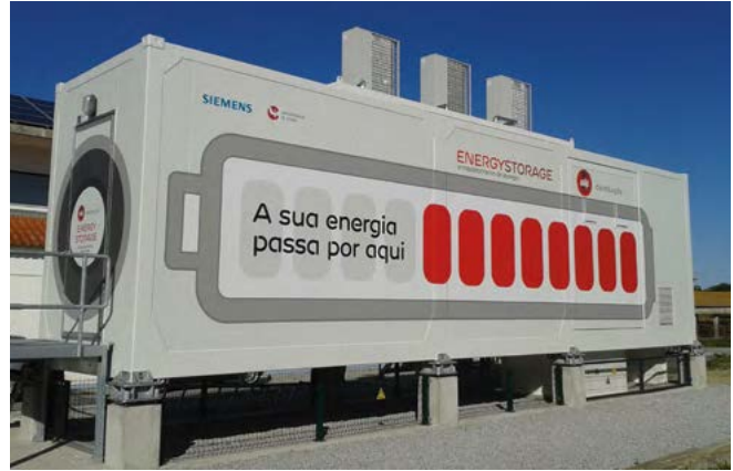
Fig. 2.3-15: Turnkey solution, fully containerized, SIESTORAGE at EDP in Portugal
