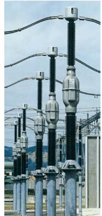
Fig. 4.2-17: 420 kV oil-paper-insulated inductive voltage transformers
