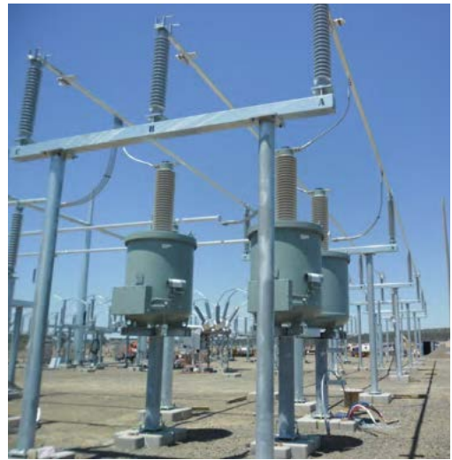
Fig. 4.2-29: 145 kV power VT for AIS
