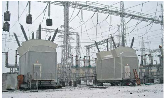
Fig. 2.4-7: 245kV E-house for Transmission utility in Siberia
