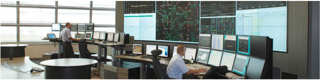
Fig. 7.1-2: Today's operator user interface of a large power control system
