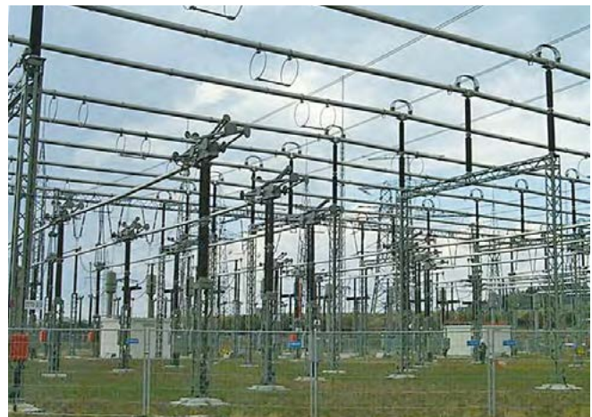
Fig. 3.1-18: Busbar disconnectors in diagonal arrangement, 380 kV, Germany
