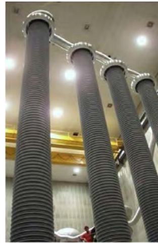
Fig. 4.2-22: Energy storage capacitor
