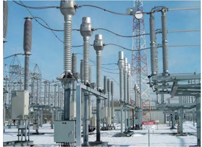
Fig. 4.2-15: 300 kV oil-immersed current transformers in Alberta, Canada
