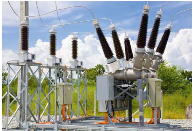
Fig 3.1-27: Dead Tank Compact (DTC)
