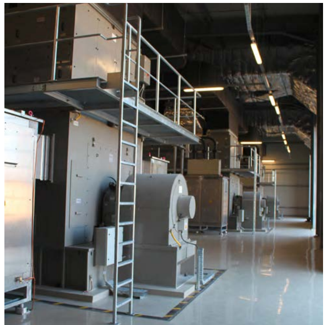
Fig. 2.2-26: Synchronous condenser building of the HVDC Black Sea Transmission Network, Georgia
