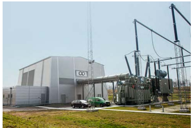
Fig. 2.2-25: Synchronous condenser in Bjaeverskov, Denmark
