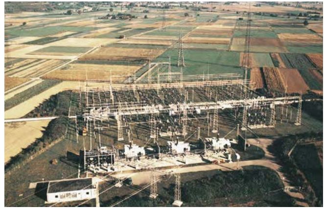
Fig. 3.1-2: Air-insulated outdoor switchgear
