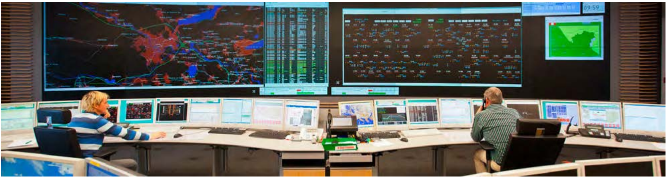
Fig. 7.1-24: Typical control room environment
