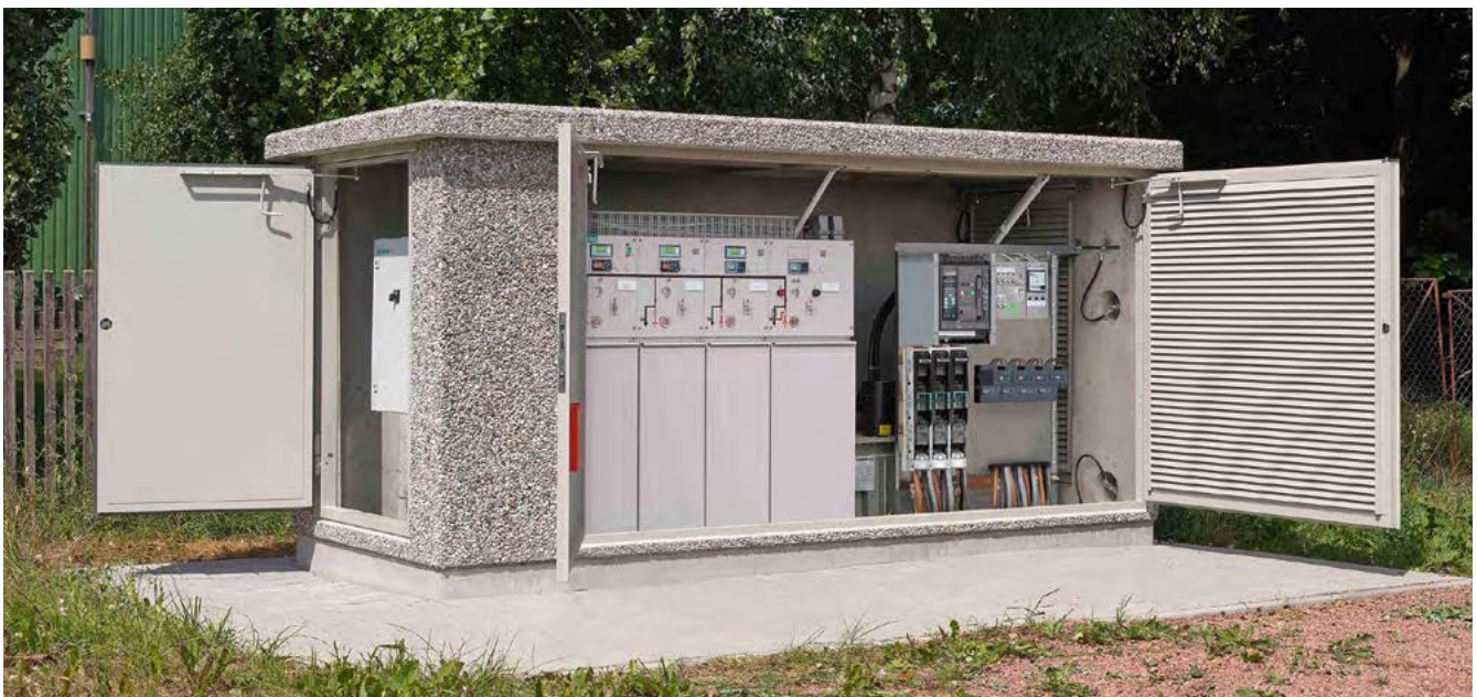
Fig. 2.6-5: Intelligent transformer substation
