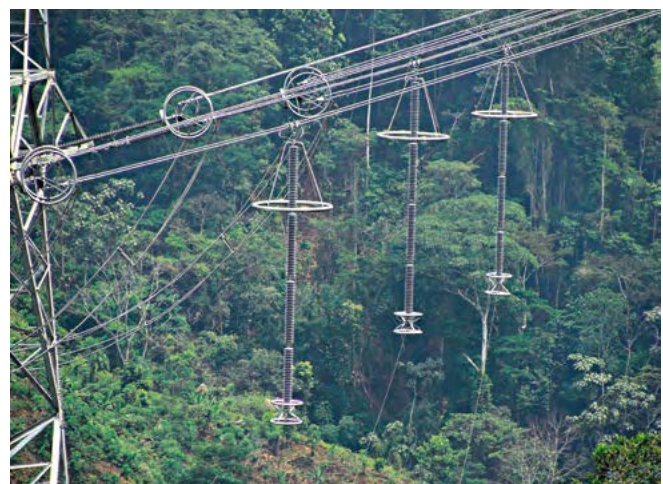
Fig. 4.2-4: 550 kV line in Colombia, NGLA solution realized with 3EL2
