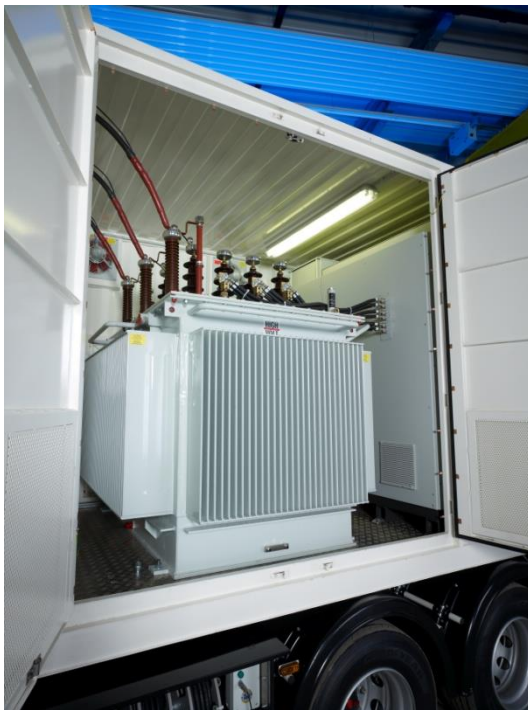
Step up transformer
