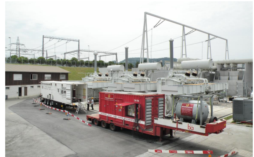
Test facility (container) and generator set
