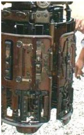
Tap-Changer after 80,000 operations
